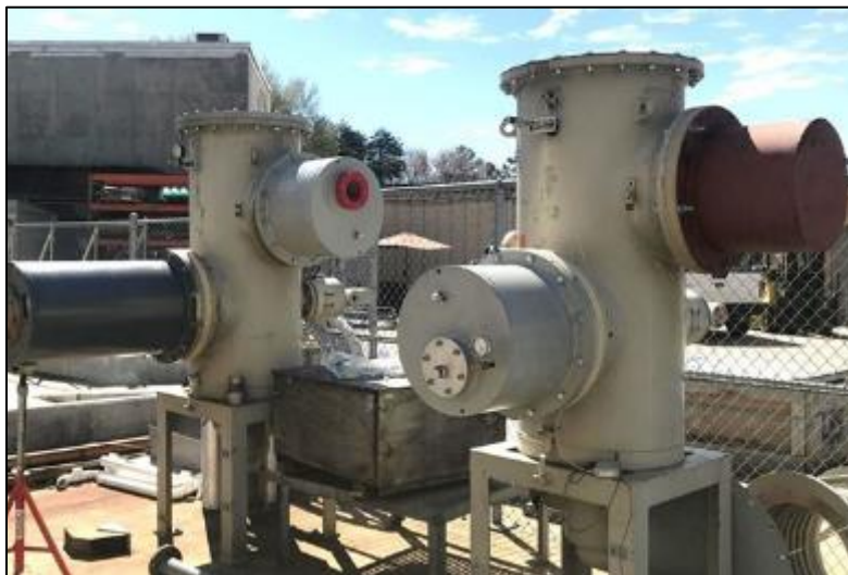
Figure 2 Outdoor Gas Insulated Equipment, EPRI GIS Lab, Charlotte, NC
