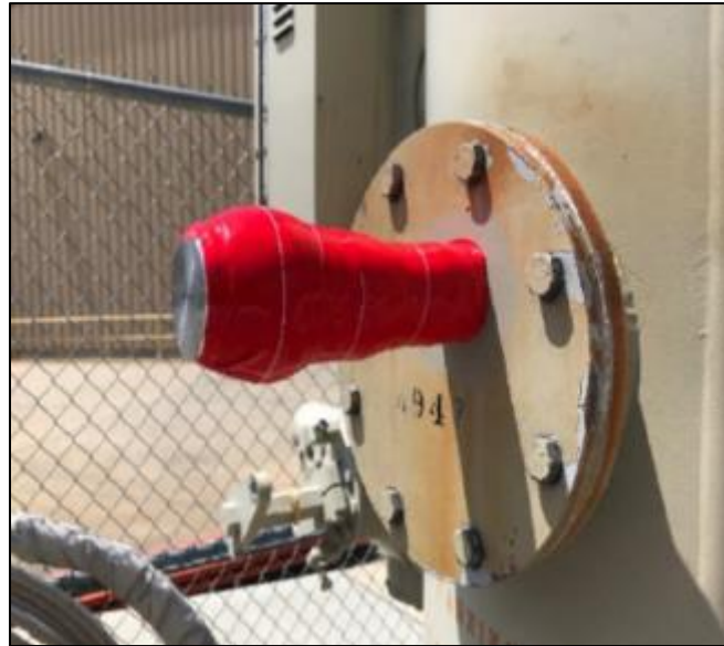
Figure 4 Leaking Threaded Fitting Sealed Using Tape and Putty
