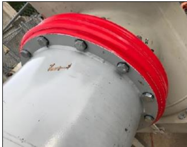
Figure 5 Leaking Flange O-ring Sealed Using Tape and Putty
