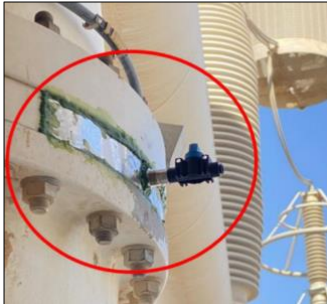
Figure 10 Leak Seal Using Patch and Adhesive
