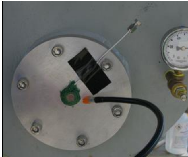
Figure 6 Leaking Bolt Sealed Using Adhesive and Vent Pipe
