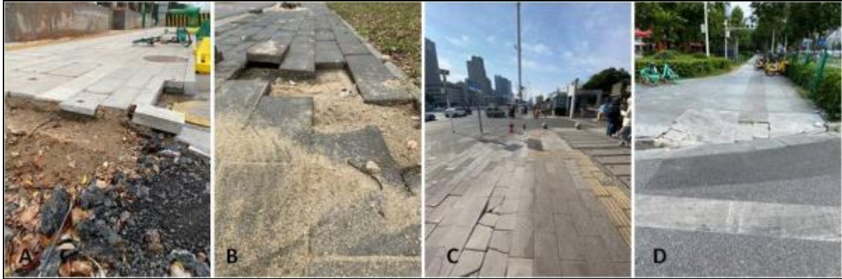
Figure 3 Walkway paving and damaged surface
