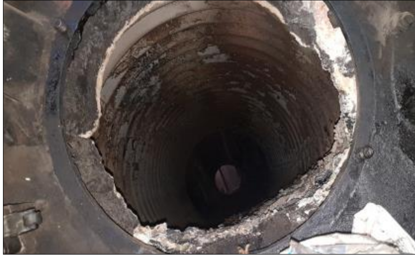
Figure 3 Real corrugated Furnace of fire tube boiler in Asmara Brewery Factory
