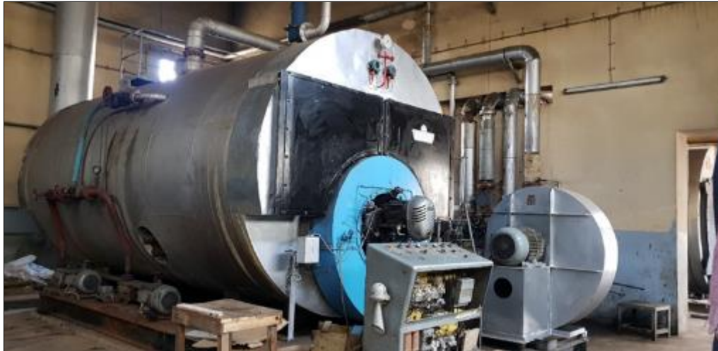
Figure 5 Firetube boiler in Asmara Brewery Factory
