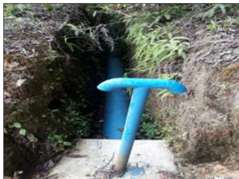
Figure 5 The condition of the pipe penstock
