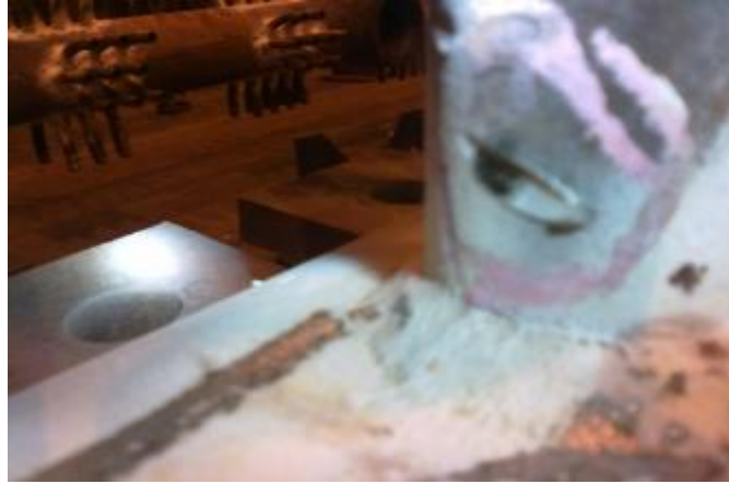
Figure 1 Tube damage due to lifting chain rubbing
