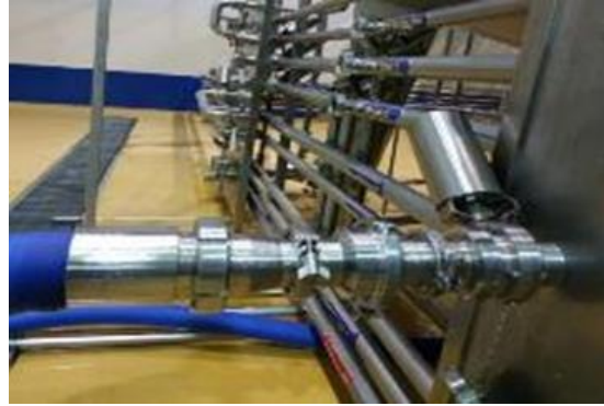
Figure 12 New setting parameter of pump system and new pipeline with diameter of 80mm
