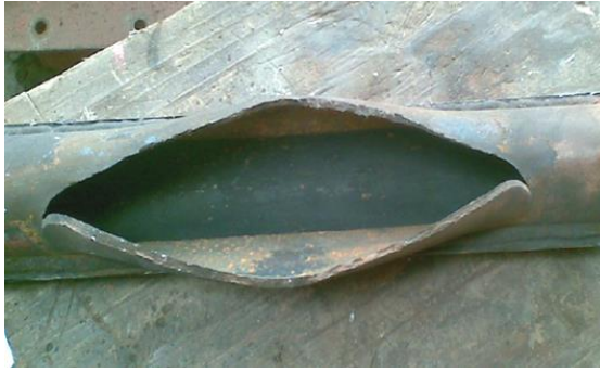
Figure 1 Ruptured boiler tube
