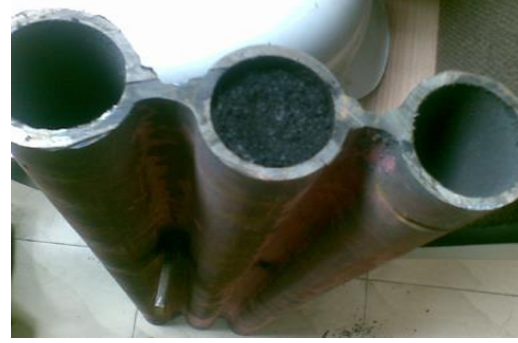
Figure 2 Blocked header tube
